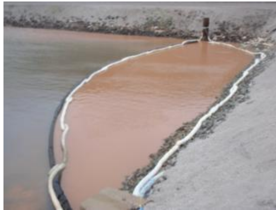
Photo 3-3: Turbid Water Escaping Around Silt Curtain
