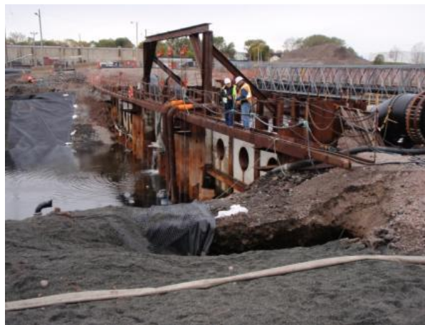
Photo 3-7: Seawater Intrusion and Collapse
