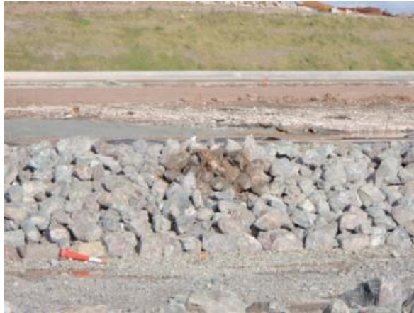
Photo 4-1: Hose Discharging Turbid Pooled Phase II Rain Water into Un-Finished Channel
