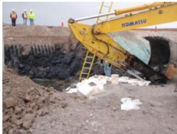
Photo 3-9: Hydraulic Oil Spill
