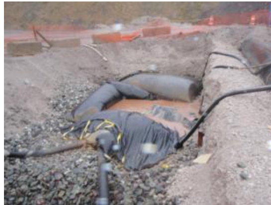
Photo 3-2: Turbid Water Flowing Through Ruptured Sediment Bags
