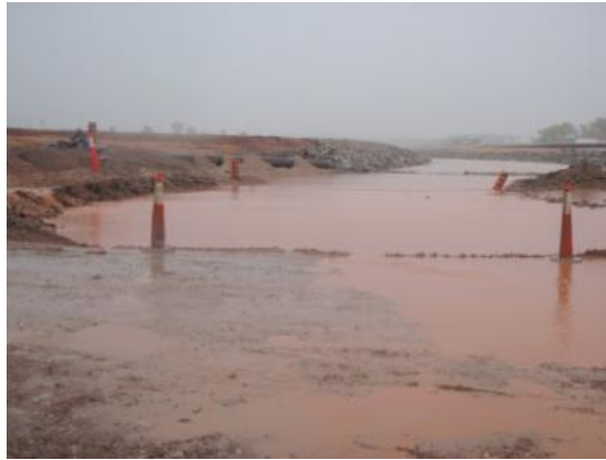
Photo 4-2: Clay-laden Surface Runoff Water Entering the Phase I Channel During Heavy Rainfall
