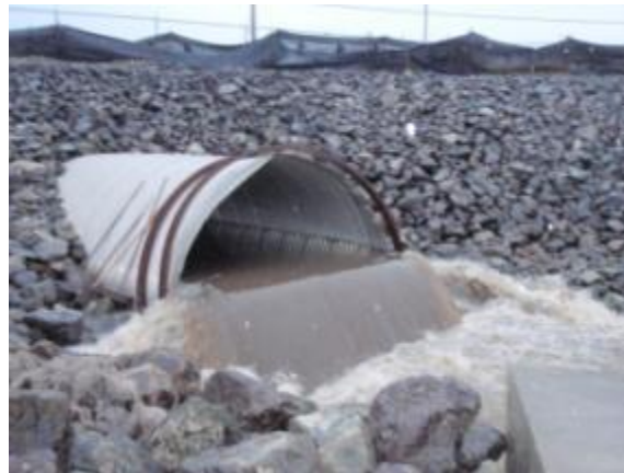
Photo 2-5: Fish Screens Breached in Coke Ovens Brook
