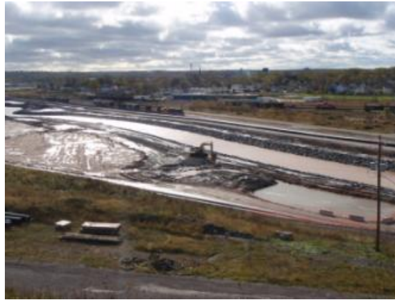
Photo 3-4: Flooding of the Phase I Channel
