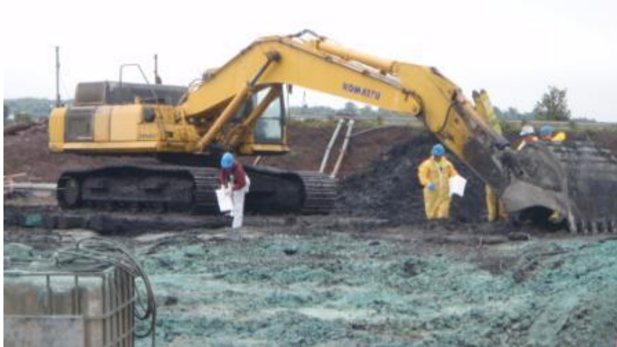
Photo 3-6: August 16, 2011 Hydraulic Fluid Leak
