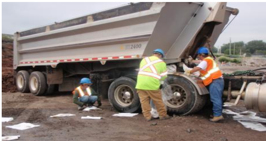
Photo 4-4: Absorbent Pads Used to Contain Hydraulic Fluid Leak
