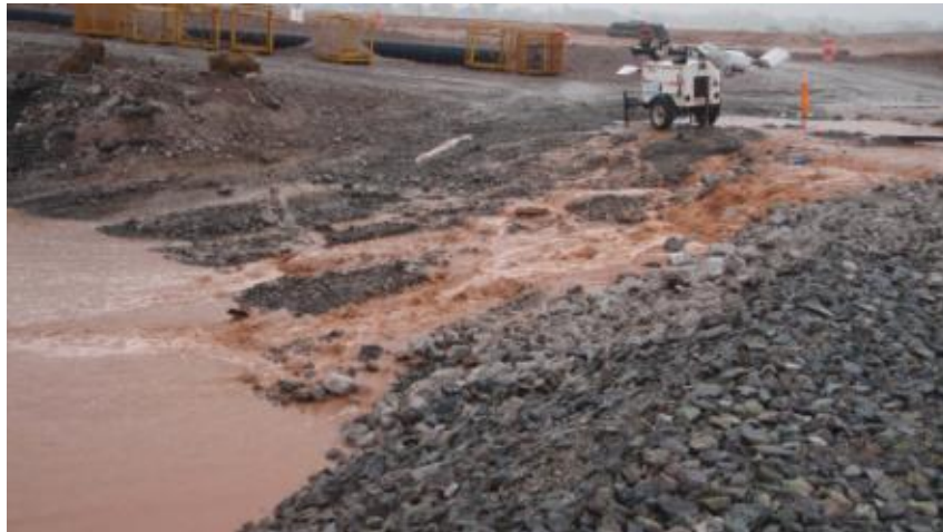
Photo 3-1: Clay Impacted Water Flowing into Ferry Street Sump
