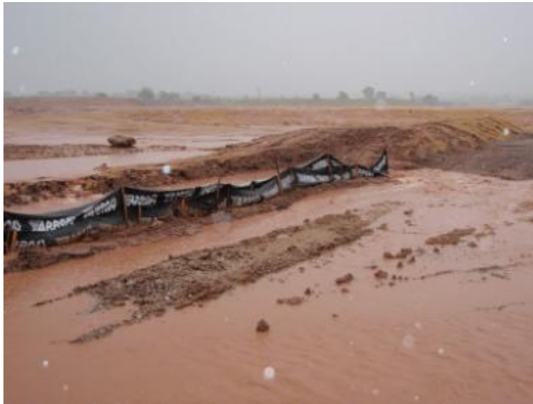
Photo 4-2: Clay Laden Water Enters TP6B Sump Area
