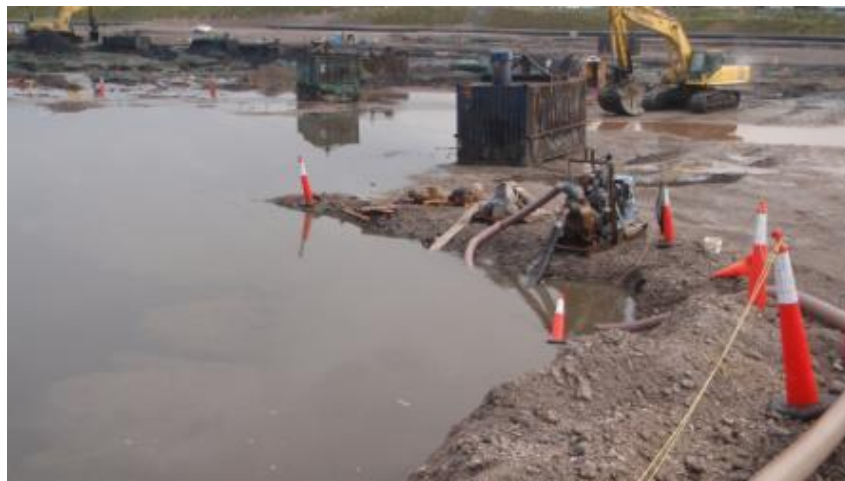
Photo 3-2: Sewage Impacted Water Overflowing the Southwest Sump
